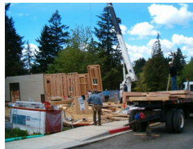
The Armstrong System at a recent home set. Sided Wall panels are lifted by a crane truck and set in place.
